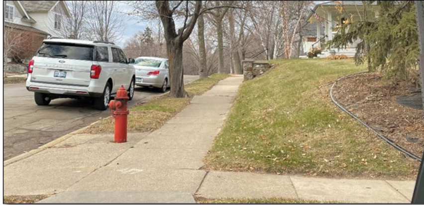
Photograph 12: Norway maple growing in Excelsior in a narrow boulevard, heaving the sidewalk adjacent near a fire hydrant
